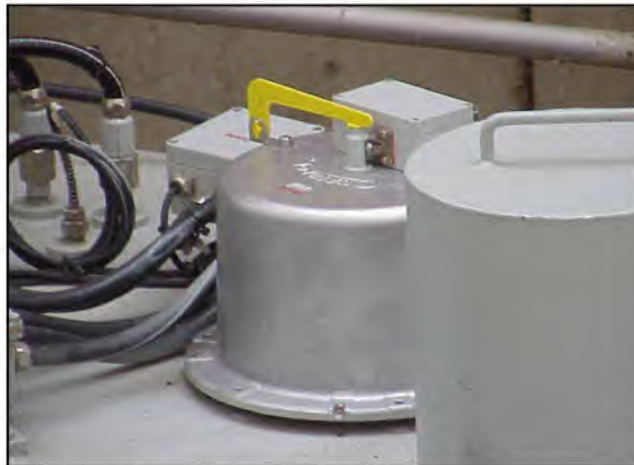
Figure 30 – Photograph of a Pressure Relief Device.
