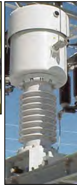
Current Transformer in Switchyard.
