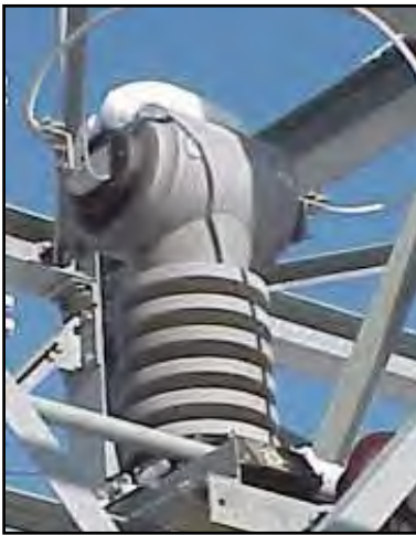
Current Transformer in Switchyard.
