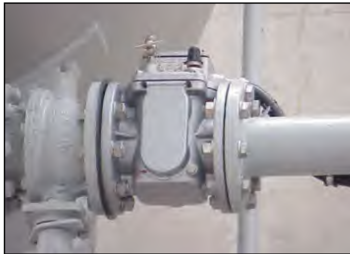
Figure 34 – Photograph of a Buchholz Relay.
