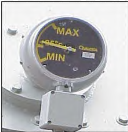
Figure 28 – Conservator Oil Level.
