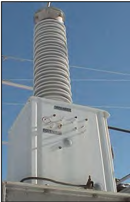
Potential Transformer in switchyard.
