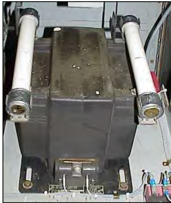
Inside Potential Transformer with Fuses.
